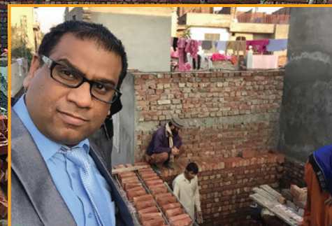
Pastor Javed Rauf, president of JCTV-Pakistan, at the new studio construction site.
